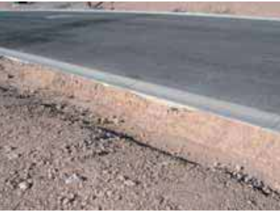
A cut-back curb is installed behind the curbline by cutting out a trench that measures about 10 to 15 cm (4 to 6 inches) deep and 0.6 to 1 m (2 to 3 ft.) wide. It is intended to collect the sediment that has eroded from the site, allowing it to settle out behind the curb instead of on the pavement.
