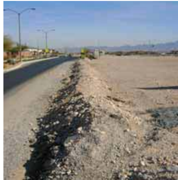
A V-ditch with a berm usually is used to retain run-off from a site. It can be a good alternative to silt fencing in low-rainfall areas. The berm is installed closest to the project. The V-ditch, used to collect any sediment from the berm, is dug on the perimeter side of the berm.
